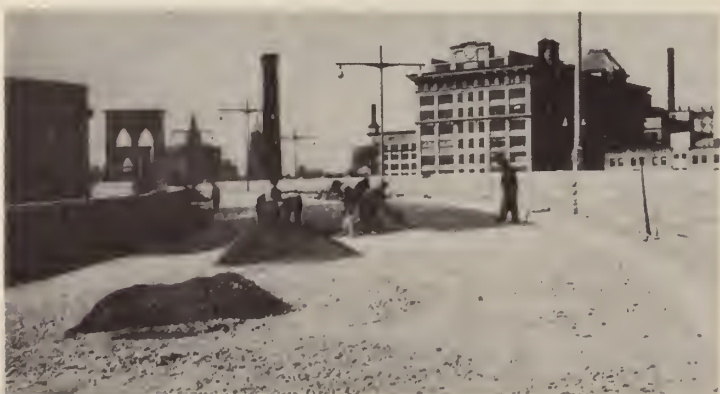
Temporary paving, to allow for settling of the fill, is laid on north roadway approach.
